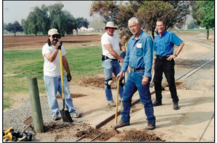
9. New cement road crossing on the Vandenberg Extension, left to right Paul Lavacot, Mike Gardner, John Noble and Phil McFadden. March 24, 2001
