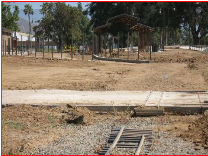
Looking from the end of our work-progress, towards the new Iowa Station: We’re really close, folks!
